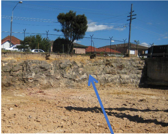
Rock face had to be cut back and stabilised to install hardstand area
